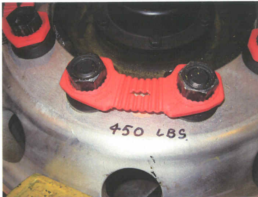
Figure 12 : Sample 10-03-C0152-10 installed on 450 ft-lb torque nuts
